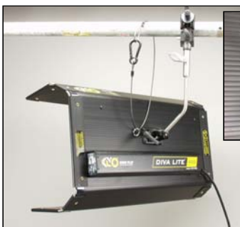
Mounted to pipe grid
